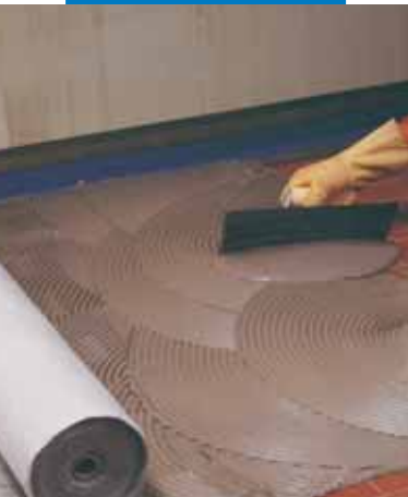
Application of the first layer of Mapelastick, and successive laying of Mapetex Sel
