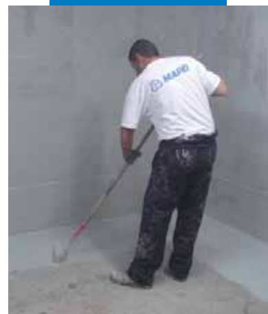
Mapelastic Foundation spread on by roller to waterproof against water in counter pressure
