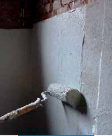
Application of Mapelast ic Foundation by roller on a substrate evened out using Planitop HDM Maxi
