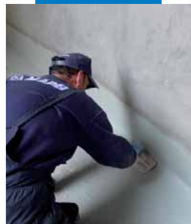
Mapelastic Foundation spread on by trowel to waterproof against water in counter pressure
